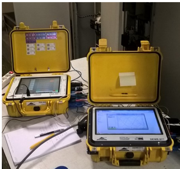
Figure 8.1: Power quality analyzers (ELCOM PNA560 and PNA571) installed in the HV substation of the steelworks.
